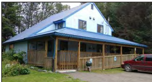
Annual maintenance to the Annex, an older, former residential building that houses several SPBHS programs, often exceeds SPBHS' entire agency maintenance budget.
