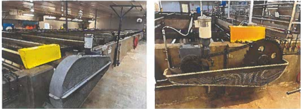
Figure 1: Clarifier 1 Upper Collection Mechanism (left) and Clarifier 2 Upper Drive Mechanism (right)
