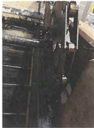
Figure 2: Clarifier 2 Southeast Sprocket and Damaged Drive Chain
