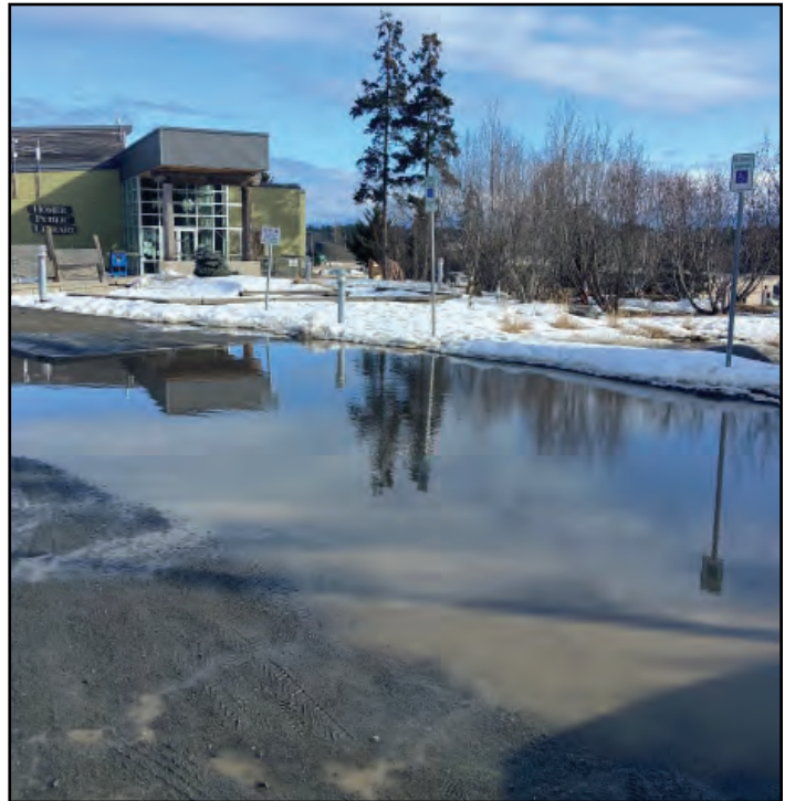
Drainage issues, especially during freeze thaw cycles in the winter and spring months create hazardous access conditions at Homer Public Library.
