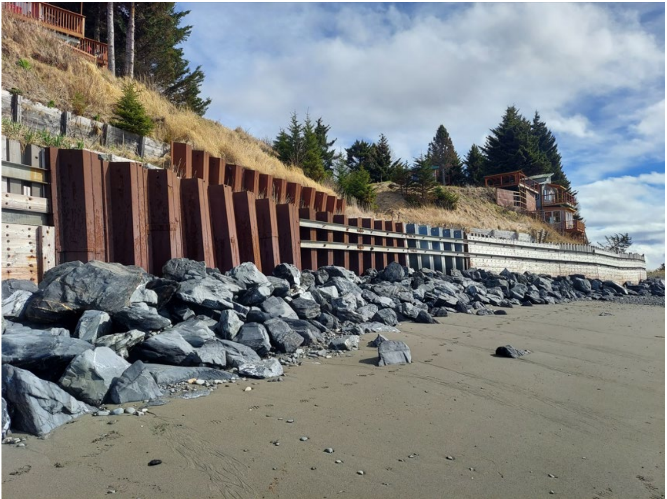
This photo shows a larger sheet pile repair that was done to strengthen up a sheet pile wall failure.
