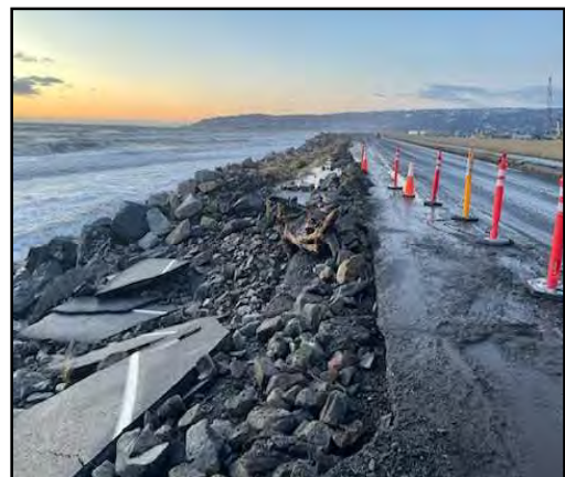
2024 erosion damage triggering disaster declarations.
