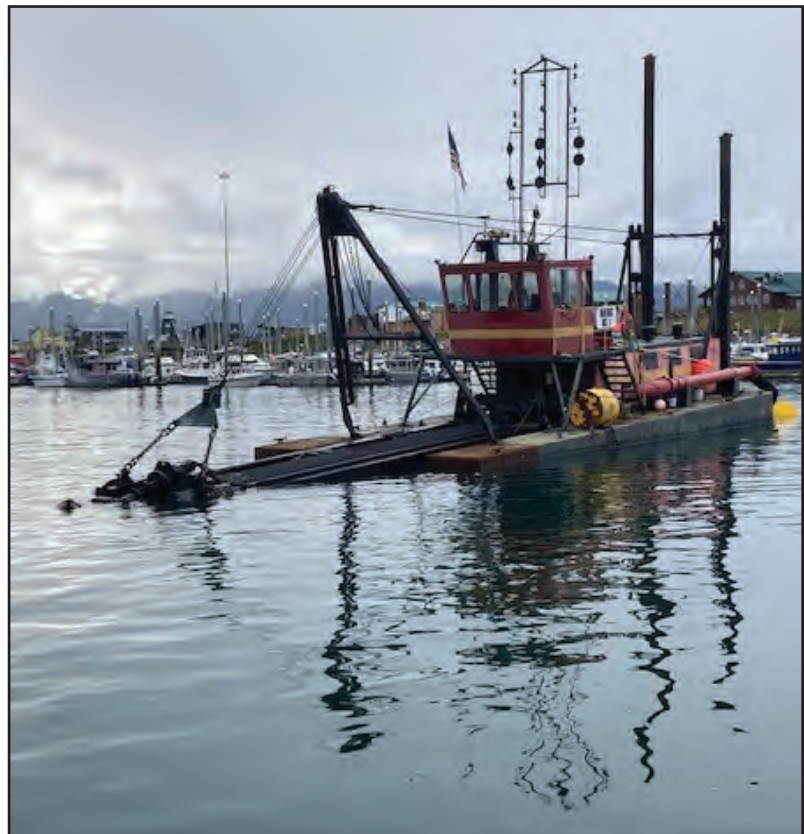
A dredge in Homer Harbor during the US Corps of Engineer's annual dredging of the harbor's navigable channel.
