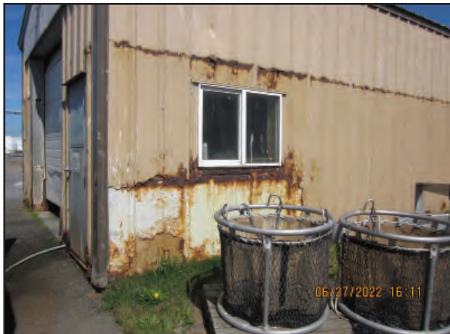
Corrosion is compromising the Fish Grinding building’s structural integrity and degrading interior fixtures.
