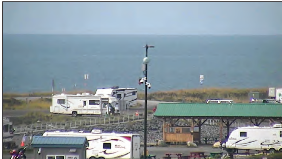
Security cameras, pictured here, center, allow harbor officers to gain situational awareness before responding to an event, to verify details of recorded events and monitor progress of evacuations or check on inundation during tsunami events.
