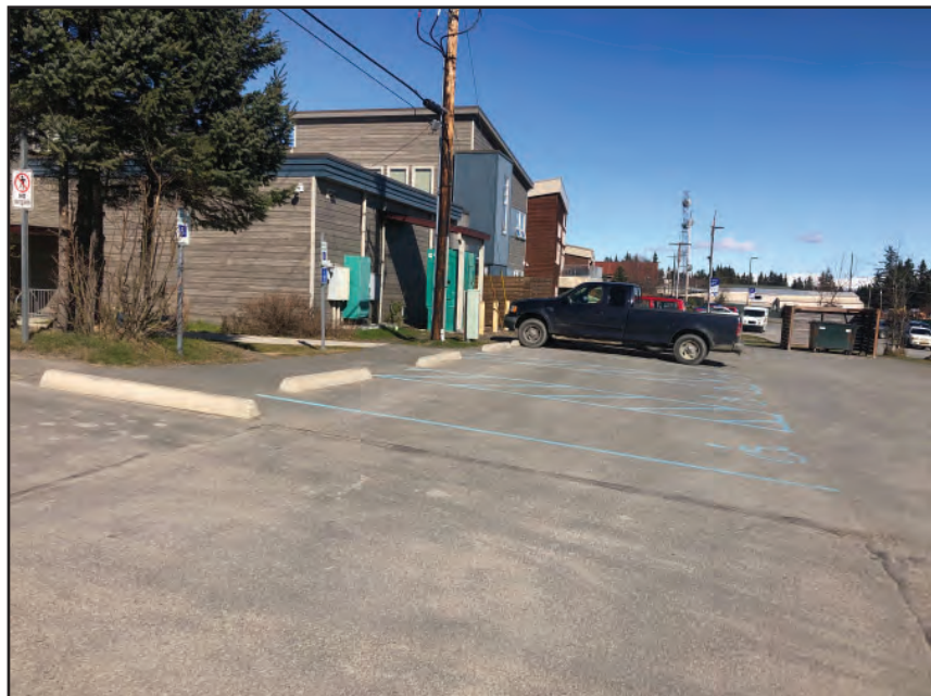
The cross slope of the accessible parking spaces at the lower entrance to City Hall exceeds the maximum allowed 1:48 under ADA standards.
