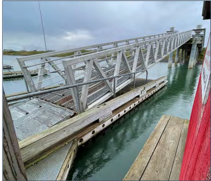
Figure 2.35: Ramp 5 trestle and gangway. Note landing on concrete float with reduced freeboard.
