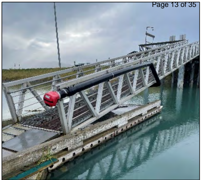
Figure 2.13: Fire system HDPE piping on Ramp 4.
