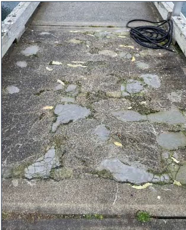
Figure 2.39: Deteriorated/patched concrete on main floats.
