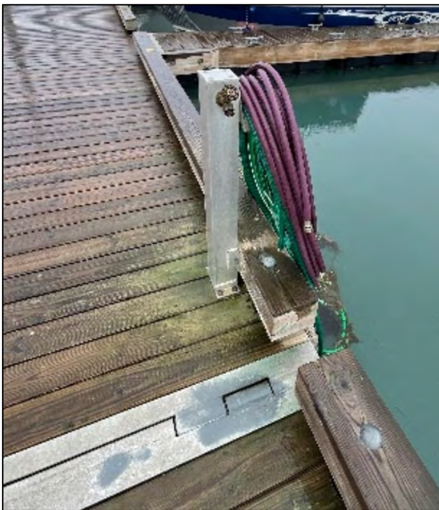
Figure 2.10: Hose bib riser, typical on R & S Floats. Note fungal growth on timber and partially worn anti-skid on steel hinge connections.
