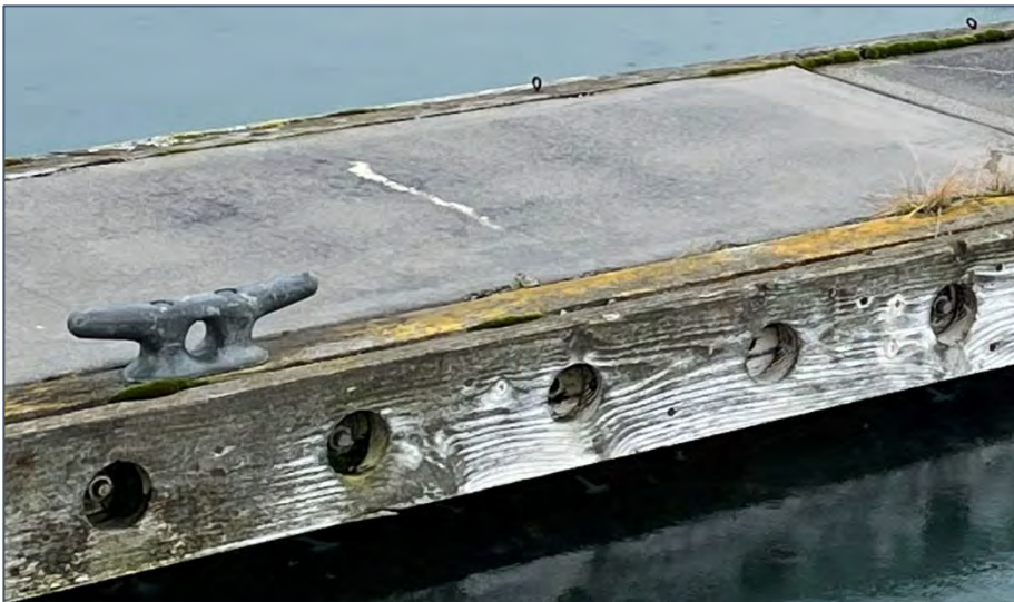
Figure 2.37: Through rods corroded or missing.
