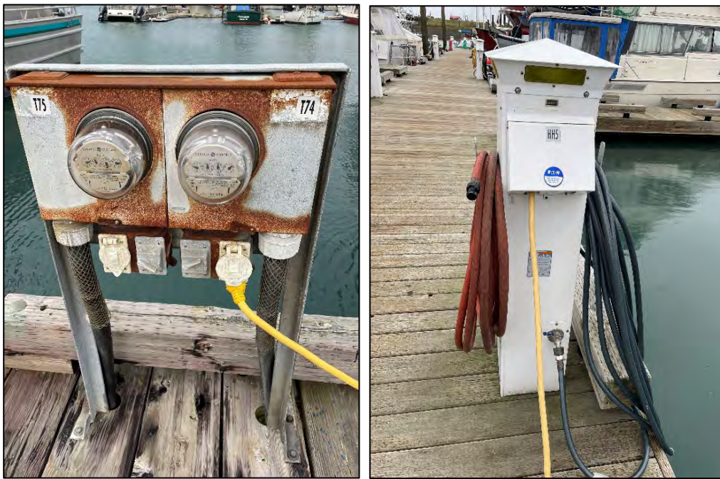
Figure 2.55: Electrical power service pedestals on EE Float (left) and typical of HH & JJ Floats (right). Note that the newer pedestal also incorporates water hose bibs.
