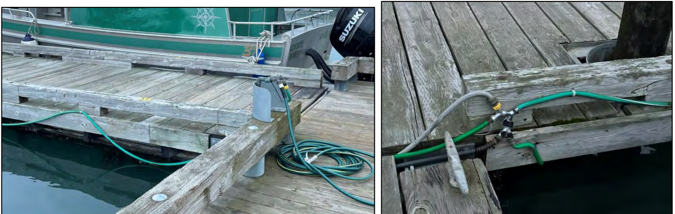
Figure 2.54: Typical water service to main floats provided from headwalk float by various hoses/connections.
