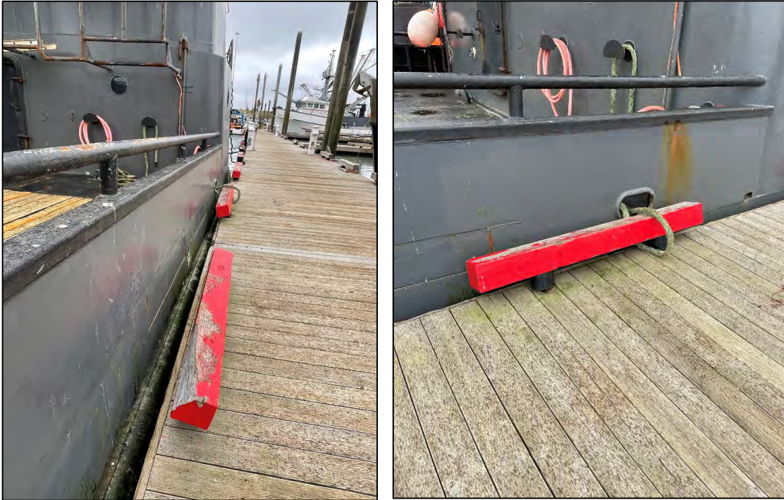
Figure 2.53: Example of several bullrails that have been damaged on JJ Float.
