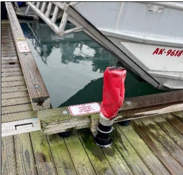
Figure 2.12: Fire suppression system standpipe/hydrant near J Float
