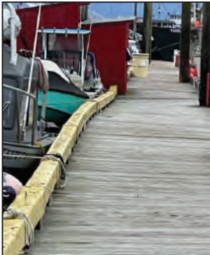
The Headwalk Float AAA is warped, suggesting a failure in the structural members below the deck and lack of flotation..
