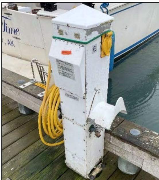
Figure 2.18: Power/water pedestal coating damage
