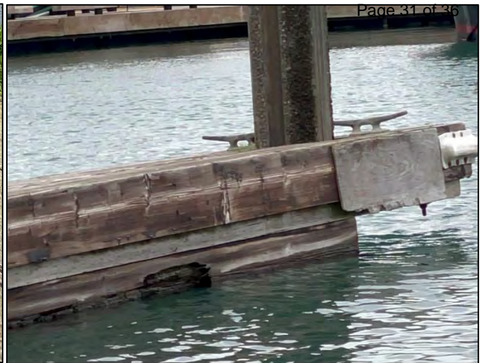
Figure 2.50: Example of a listing stall float (GG Float). Also note advanced rot/deterioration of below-deck timber.
