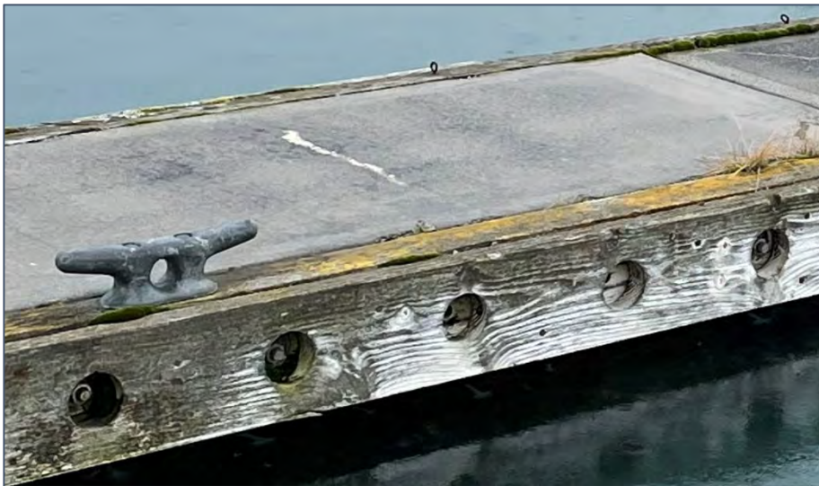
Figure 2.37: Through rods corroded or missing.
