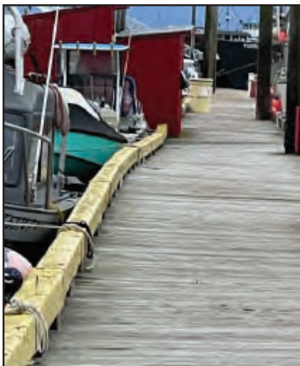
The Headwalk Float AAA is warped, suggesting a failure in the structural members below the deck and lack of flotation..
