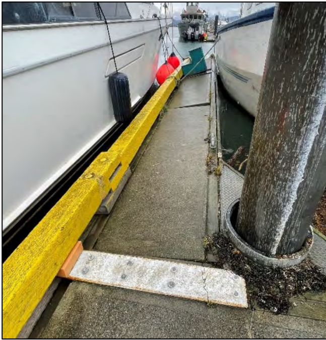
Figure 2.30: A metal plate has been installed to a broken Tee Float. Note the bullrail has come apart at the splice.
