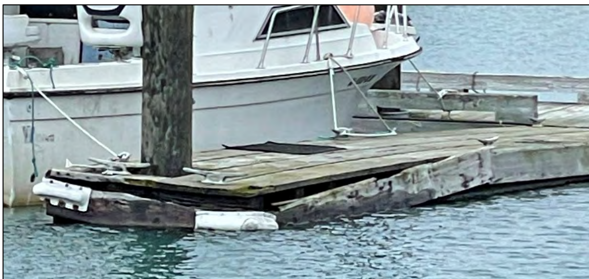
Figure 2.43: Stall Float on CC Float with damaged timber waler, rubboard, and decking.
