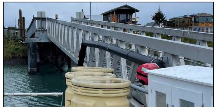
Figure 2.17: HDPE fire suppression piping at Ramp 2
