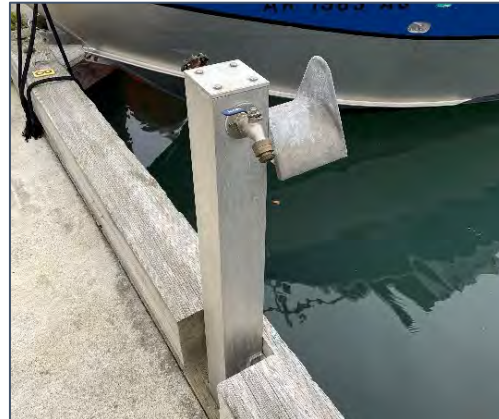
Figure 2.42: water hose bib and hose stand.
