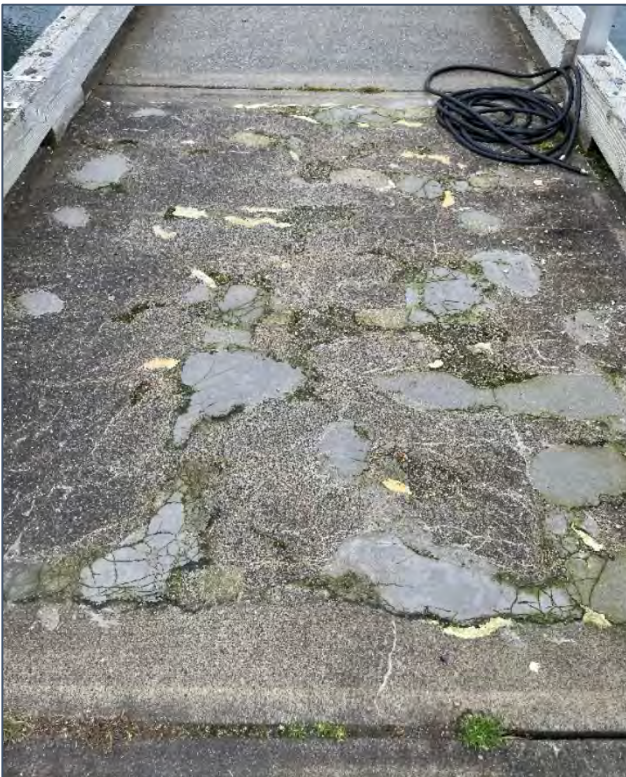
Figure 2.39: Deteriorated/patched concrete on main floats.
