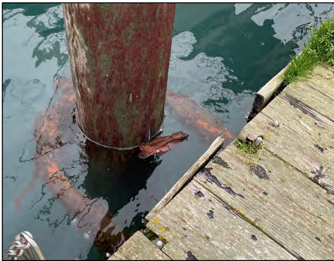
Figure 2.49: Low freeboard resulting in submerged pile collar. Also note hardware connections protruding through decking.
