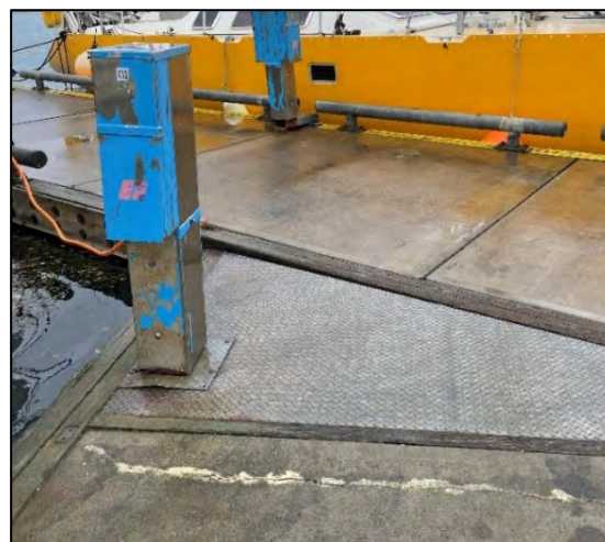
Figure 2.24: Typical power pedestal, many with damaged mounts. Note also typical minor crack in concrete.
