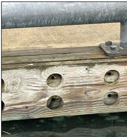
Figure 2.22: Missing through rods.
