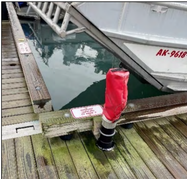
Figure 2.12: Fire suppression system standpipe/hydrant near J Float
