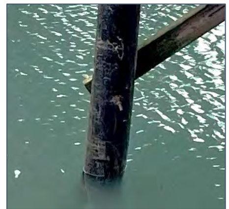
Figure 2.3: lower hardware connections appear corroded.
