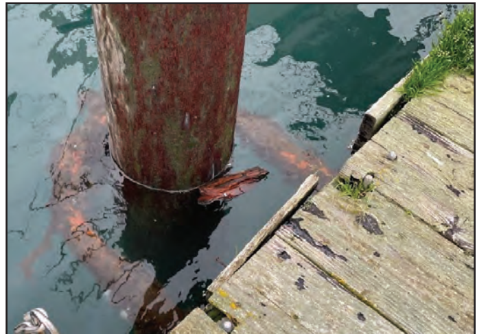
Low freeboard resulting in submerged pile collar. Decking has rot and hardware connections protrude through it.
