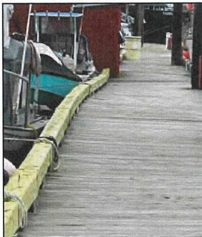
The Headwalk Float AAA is warped, suggesting a failure in the structural members below the deck and lack of flotation..
