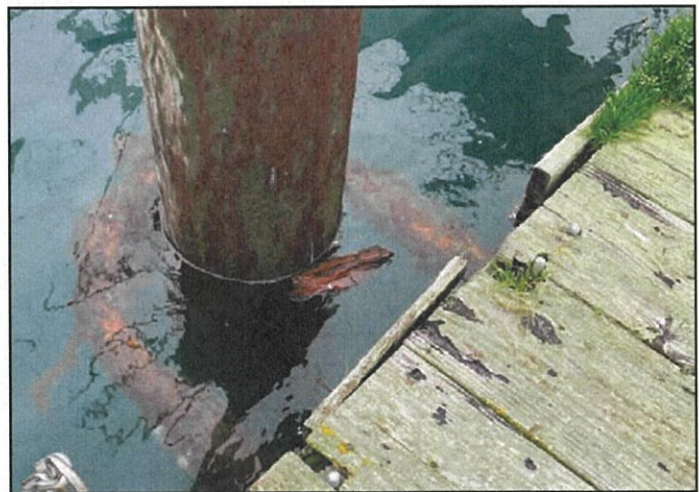
Low freeboard resulting in submerged pile collar. Decking has rot and hardware connections protrude through it.
