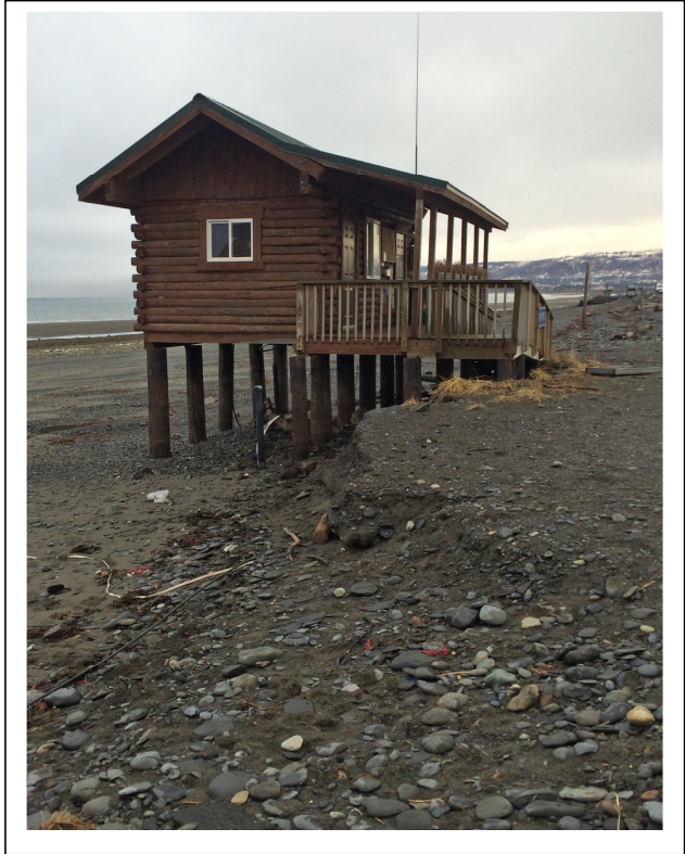
Above: In the fall of 2015, the City had this camp host building removed from the west side of the Homer Spit. Previous attempts to reduce the impact of coastal storms were not successful.
