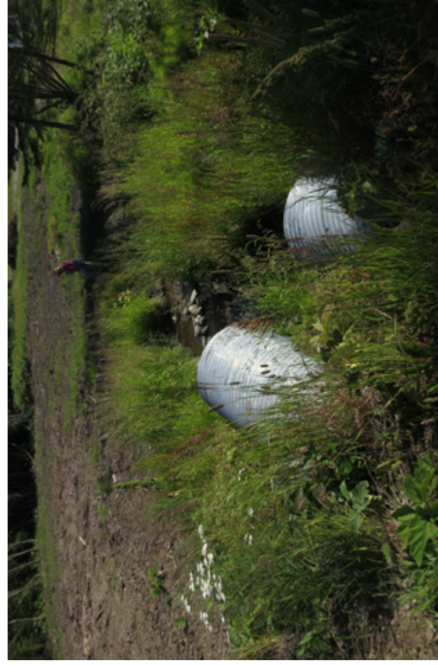
Pioneer Avenue culvert outlet. Source: Lisa Holzapfel.
