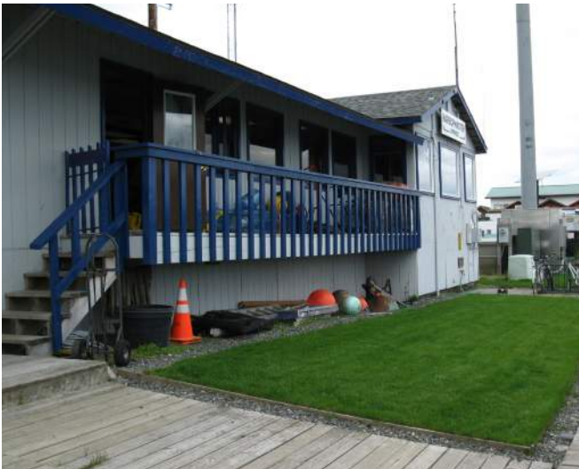
The Harbormaster's office is in poor condition, is expensive to heat, and has limited parking.
