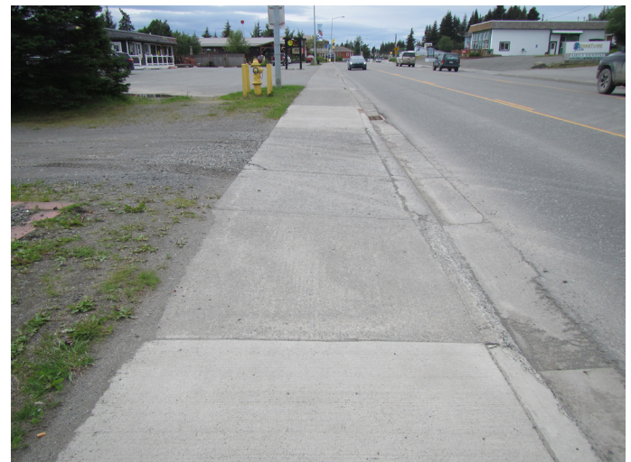
Figure 20: Driveway Entrance with Steep Cross Slope
