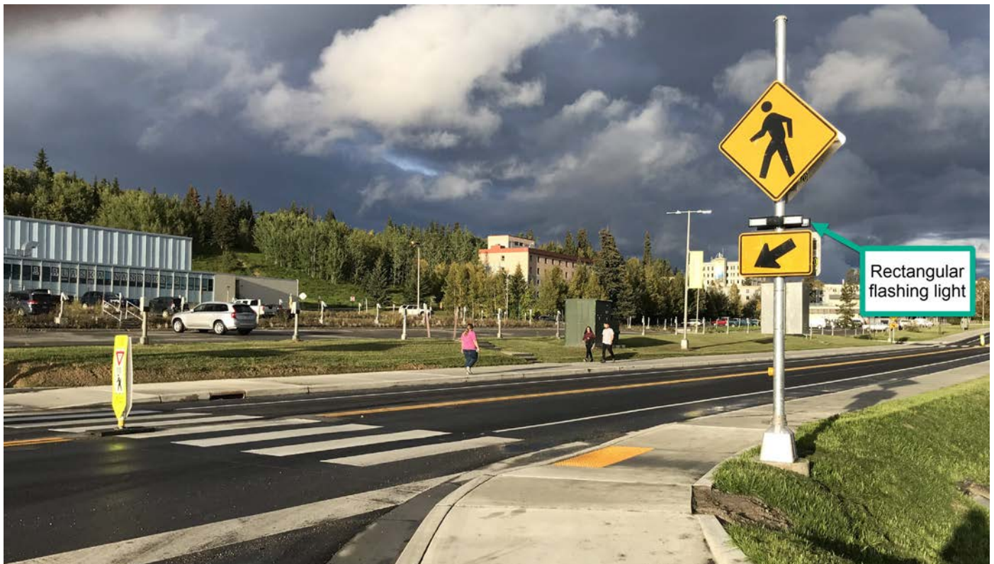
Figure 21: Electrical Warning Devices (Rectangular Rapid Flashing Beacon, or RRFB) on University of Alaska Fairbanks Campus
