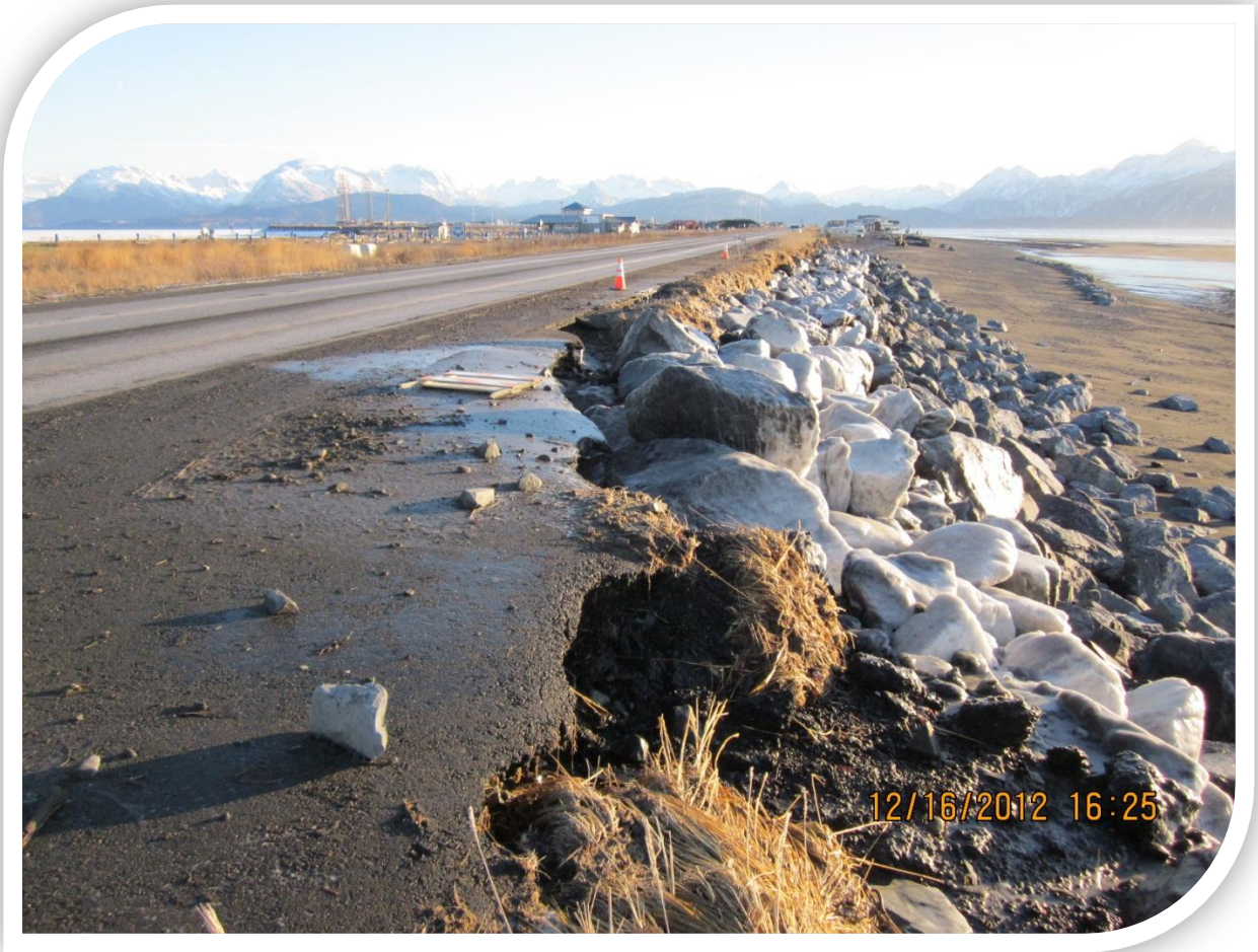
Homer Spit Road Damage from December Storms
