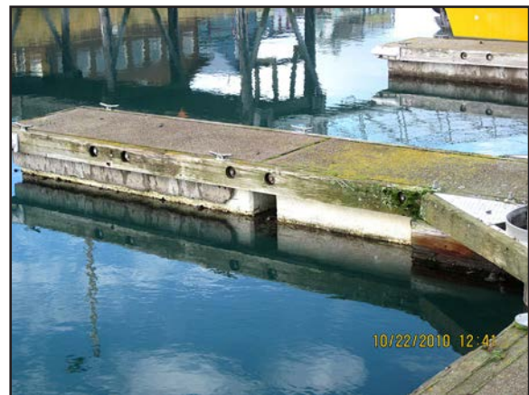
Exposed flotation on a damaged float.
