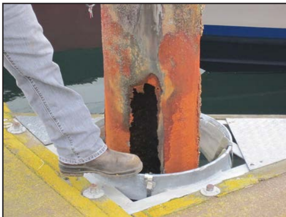
Hole in damaged piling that needs replacing
