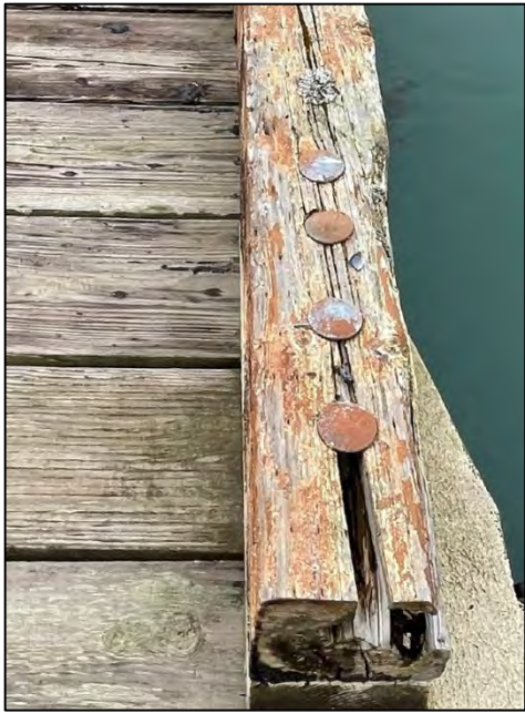
Figure 2.44: Cracked and deteriorated bullrail
