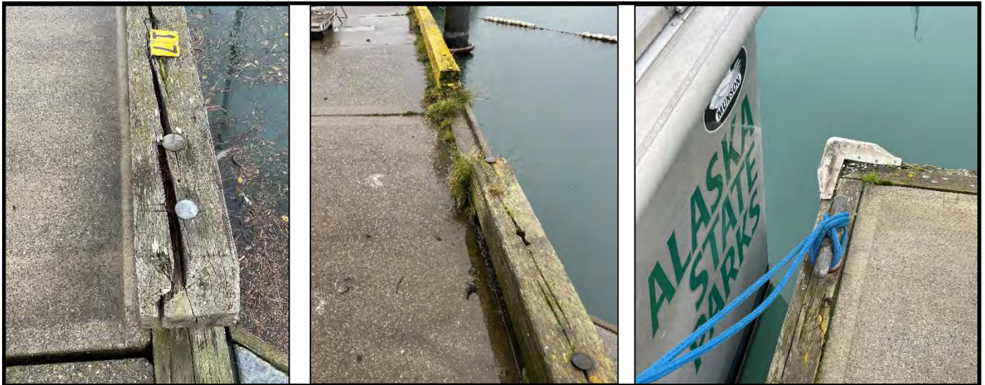
Figure 2.28: Bullrails will major splits and missing section, and cleat mounted in damaged timber waler.
