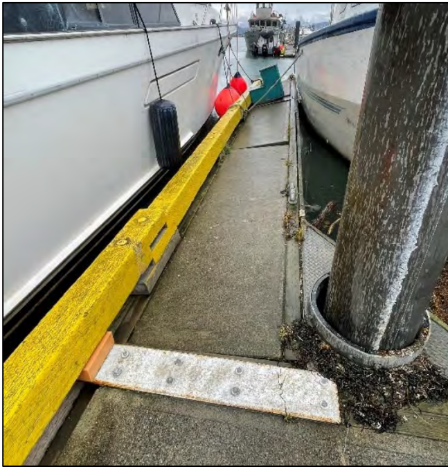
Figure 2.30: A metal plate has been installed to a broken Tee Float. Note the bullrail has come apart at the splice.
