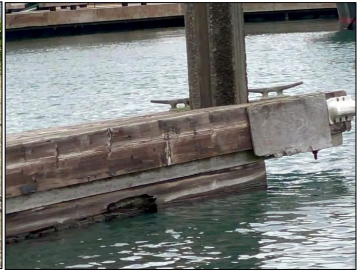
Figure 2.50: Example of a listing stall float (GG Float). Also note advanced rot/deterioration of below-deck timber.
