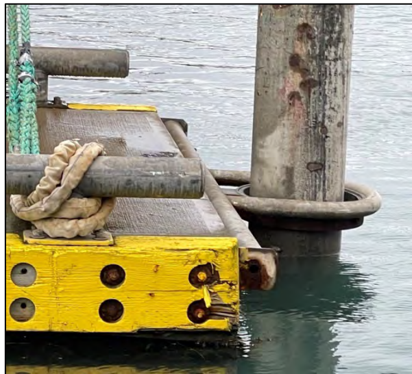
Figure 2.23: Pit corrosion and other areas of active corrosion is evident on some piles
