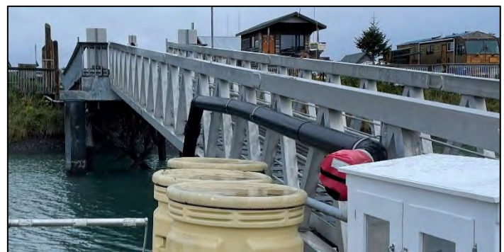
Figure 2.17: HDPE fire suppression piping at Ramp 2
