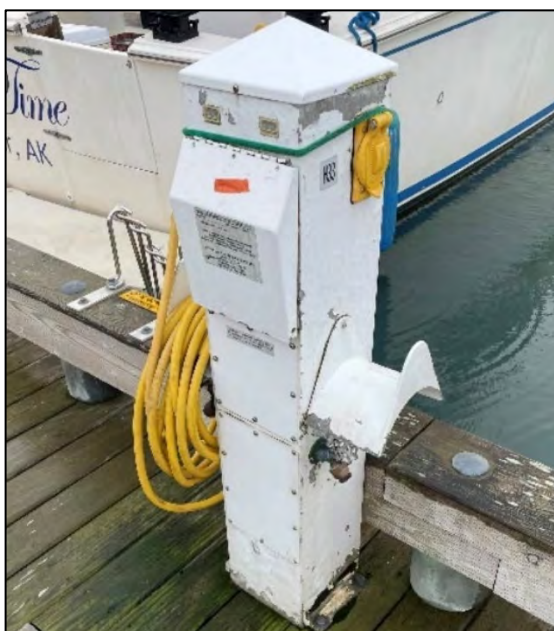
Figure 2.18: Power/water pedestal coating damage
