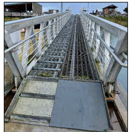
Figure 2.1: aluminum gangway with steel floor grating and landing tracks
