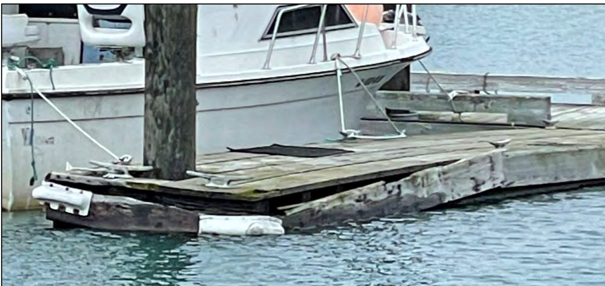
Figure 2.43: Stall Float on CC Float with damaged timber waler, rubboard, and decking.
