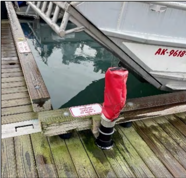
Figure 2.12: Fire suppression system standpipe/hydrant near J Float
