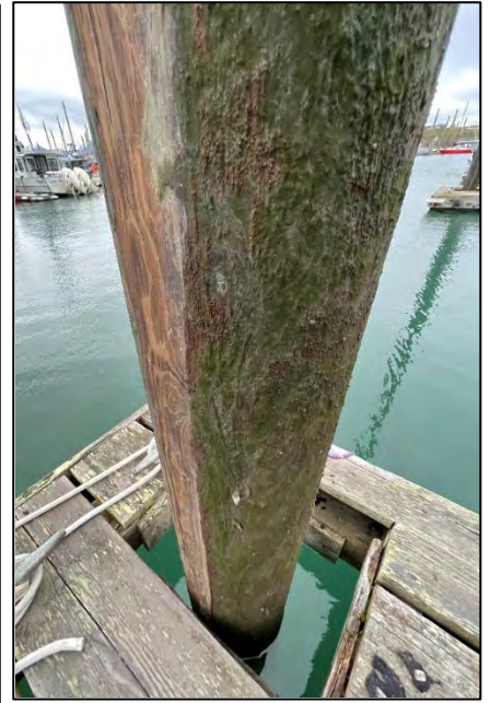
Figure 2.46: Moderate wear on timber piles.
