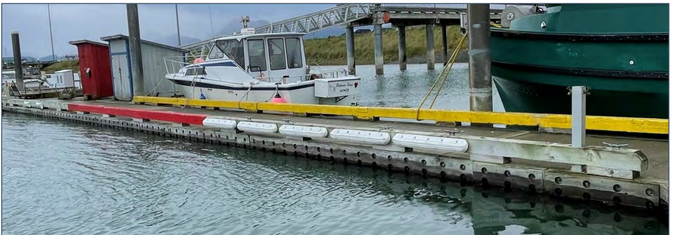
Figure 2.36: System 2 Headwalk float has reduced freeboard and appears to be listing to one side, as noted by partially submerged rubboards.
