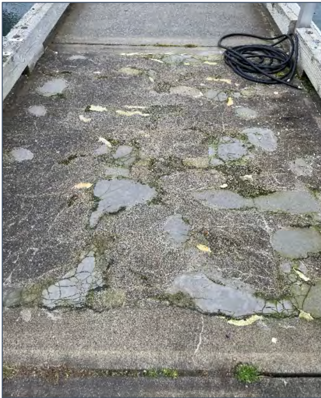
Figure 2.39: Deteriorated/patched concrete on main floats.
