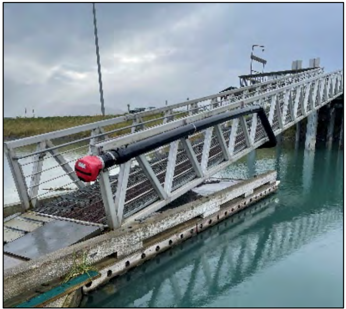
Figure 2.13: Fire system HDPE piping on Ramp 4.
