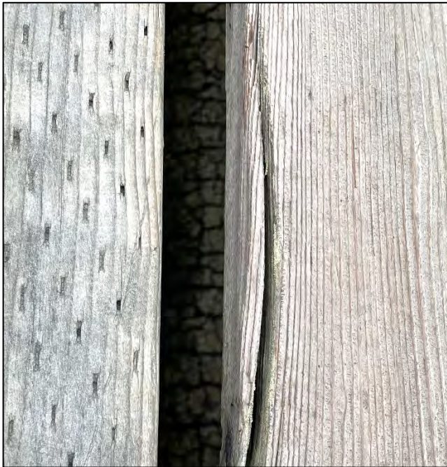
Figure 2.48: View between deck boards of deteriorated flotation foam.
