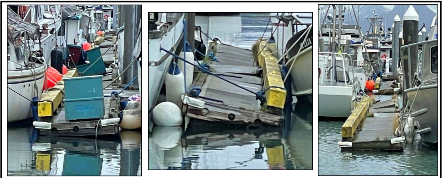
Figure 2.29: Tee floats, located along the harbor channel, are broken and severely listing.
