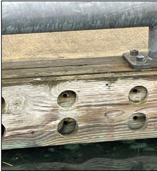
Figure 2.22: Missing through rods.
