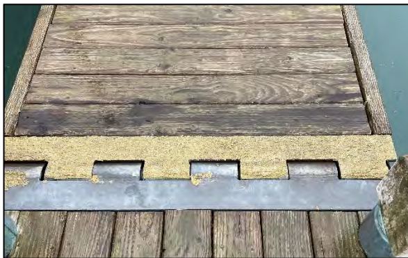
Figure 2.16: Worn non-skid coating at hinges.
