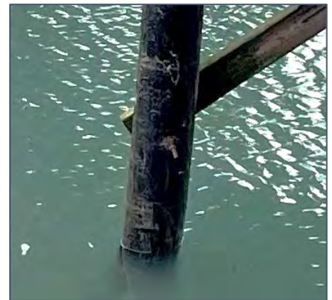
Figure 2.3: lower hardware connections appear corroded.
