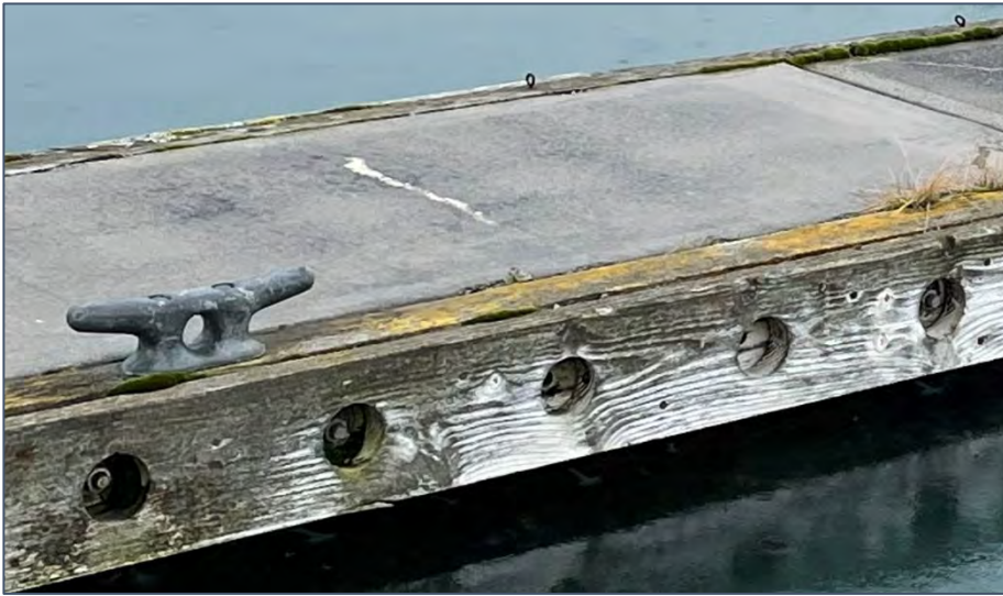
Figure 2.37: Through rods corroded or missing.
