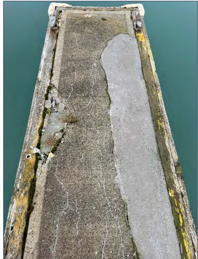
Figure 2.40: Patched concrete and deteriorated waler and rubboards on stall floats.
