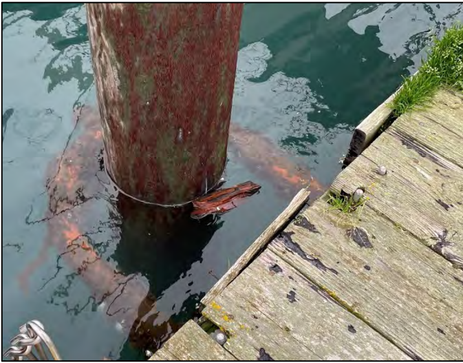
Figure 2.49: Low freeboard resulting in submerged pile collar. Also note hardware connections protruding through decking.
