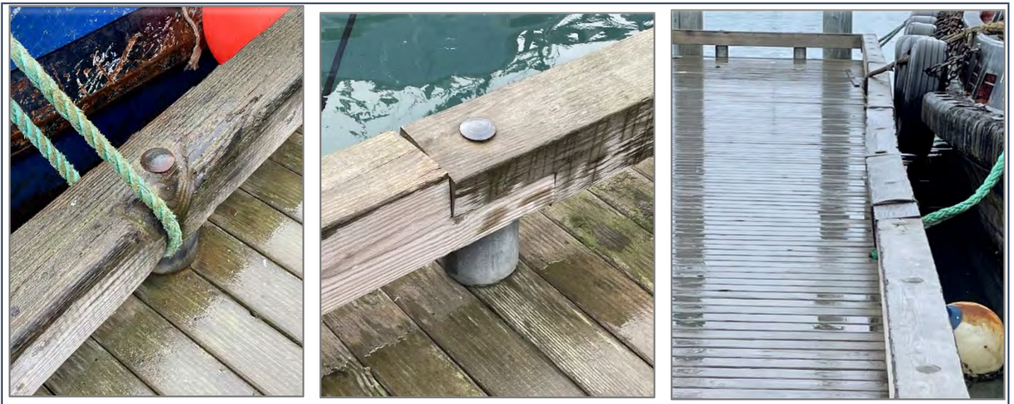
Figure 2.15: Bullrails worn, twisted out of position, and broken from supports.
