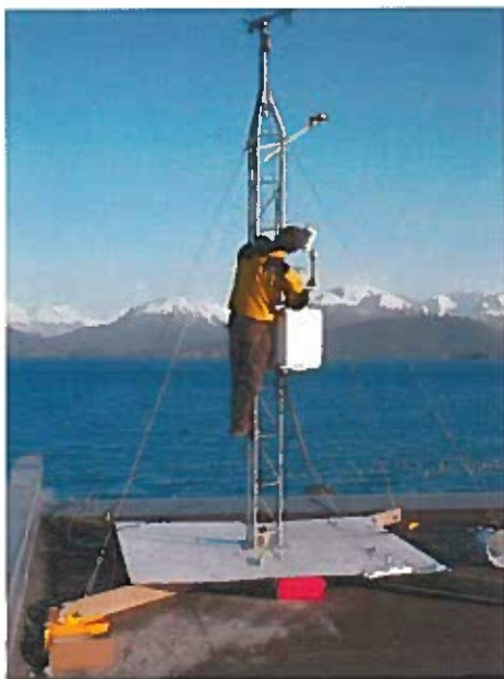
Figure 1. This photo shows the set up of a KBRR MET station on the Land's End roof top and one of our researchers accessing the tower.
