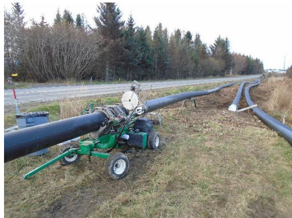
40' long, 12" HDPE water main sections being "fused" together in preparation for installation along Kachemak Drive
