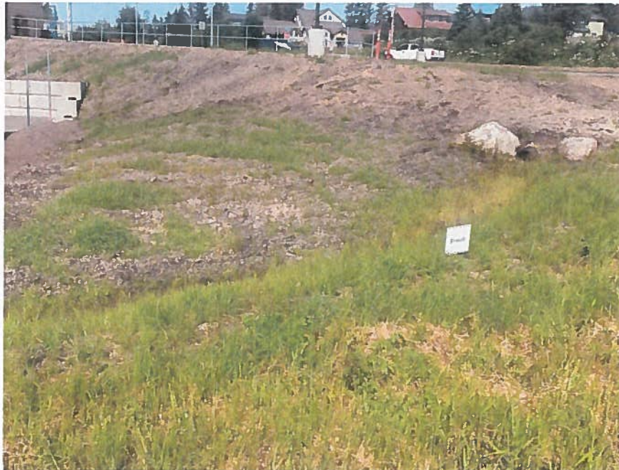
New BIOSWALE - Filters storm water runoff of sediment and pollutants
