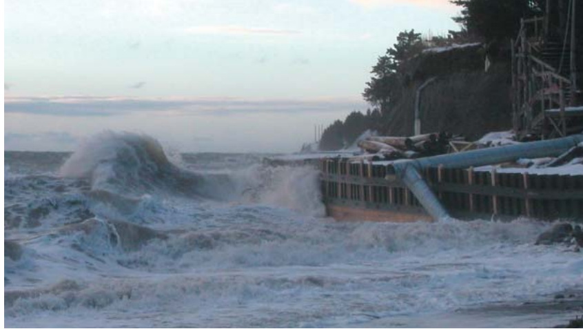
The Homer seawall was battered by waves during a winter storm when the wall was still under construction. (Photo by Carl Schoch)
